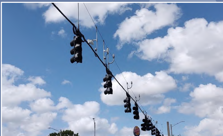
Multiple microwave radar sensors installed for span wire intersection stop bar detection. (Lake County)
