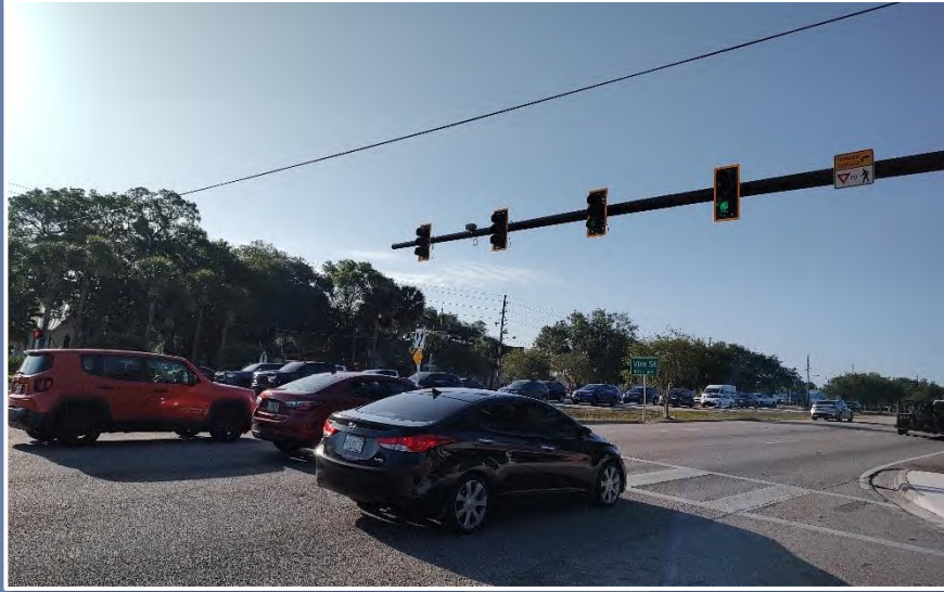
Hybrid radar-video unit installed on mast arm on the far-side of signalized intersection approach. (Osceola County)
