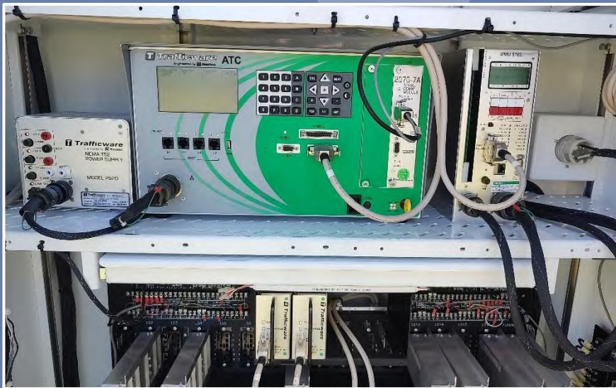
Trafficware (now Cubic ITS) ATC controller unit, NEMA TS-2, Type 1 model. (Brevard County)
