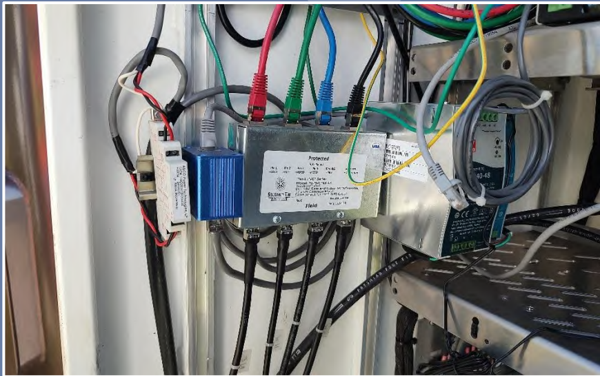
In-cabinet equipment array for hybrid radar-video unit inclusive of in-line surge protection devices and power distribution. (Osceola County).
