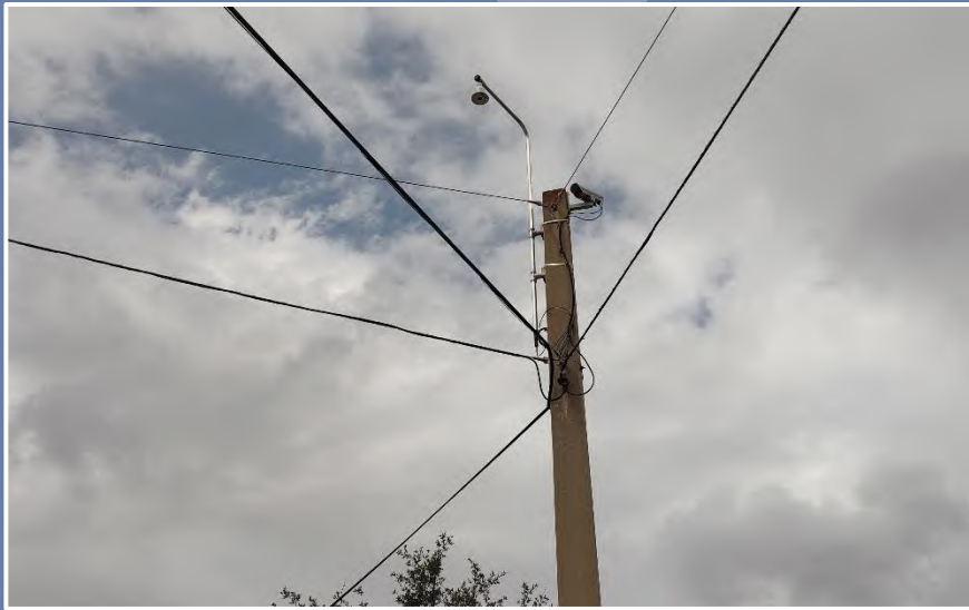
Candy cane vertical mounting arm for omnidirectional camera affixed directly to concrete strain pole for a span wire intersection. (City of Orlando)
