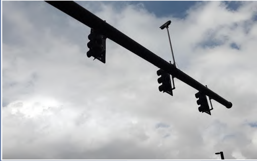
Vertical riser mounting arm installed to provide greater elevation of video detection camera above the roadway surface for advanced detection zones. (City of Orlando)
