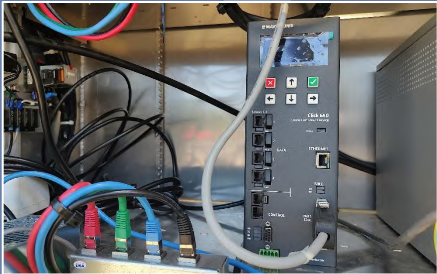
Typical in-cabinet processors for microwave sensors include embedded surge protection devices to eliminate the need for external equipment, verify with each vendor. (Orange County)
