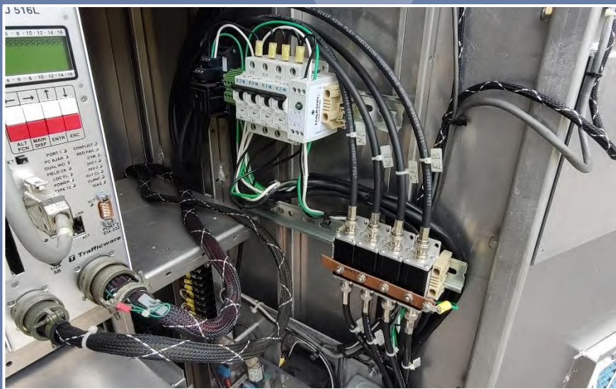
Typical in-cabinet video detection array including in-line surge protection devices, circuit breakers, and power distribution assembly. (City of Orlando)
