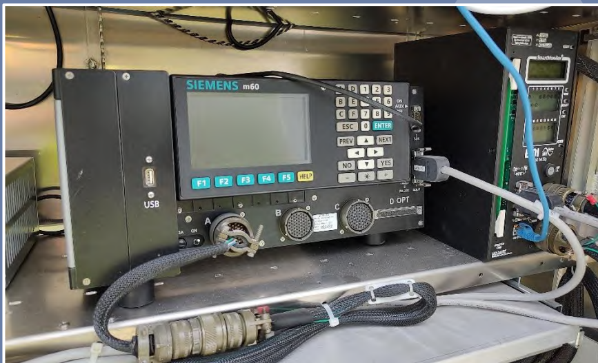
Siemens (now Yunex Traffic) m60 ATC controller unit, TS-2 Type 2 model, operated as Type 1 ("A" connector only). (Marion County)
