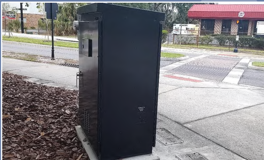
NEMA Type 6 controller cabinet assembly with matte black powder-coat finish and additional rear door. (Seminole County)
