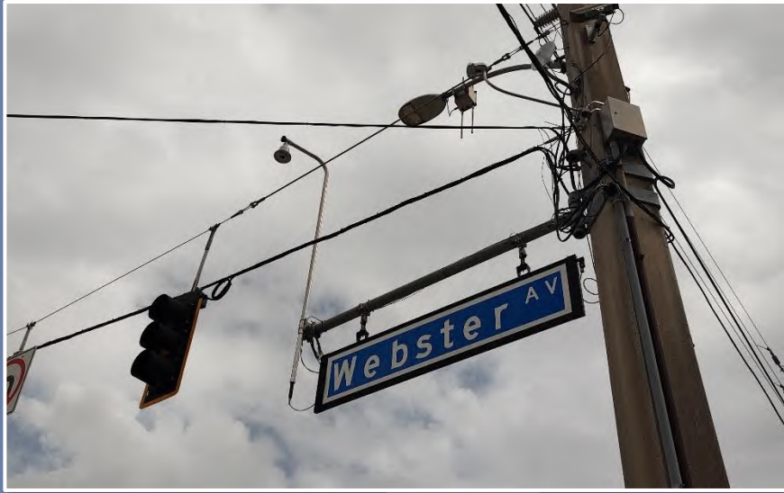
Omni-directional camera sensor installed on cantilevered mounting arm for span wire intersection. (City of Orlando)
