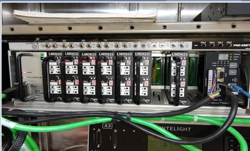
Standard detector rack with bus interface unit (BIU) and two-channel detector cards installed in controller cabinet assembly. (Orange County)
