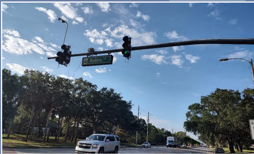
Hybrid video-radar sensors provide the ability to capture both stop bar and advanced detection zones for a single approach simultaneously. (City of Orlando)
