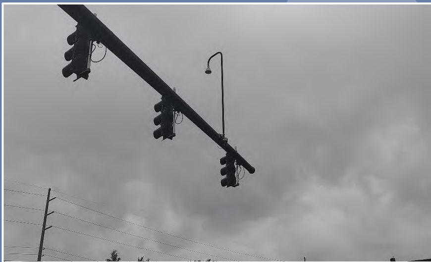
Mast arm structure with omnidirectional camera sensor positioned towards the center of the signalized intersection. (Seminole County)
