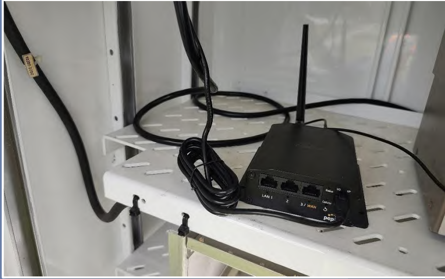
Shelf-mounted cellular modem acting as router to provide network connection between the controller and local maintaining agency network. (Lake County)
