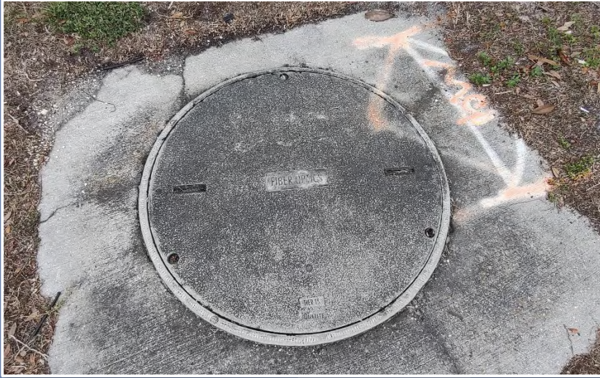
Typical round fiber optic splice vault (36" diameter) installed at the base of the controller cabinet assembly. (City of Orlando)
