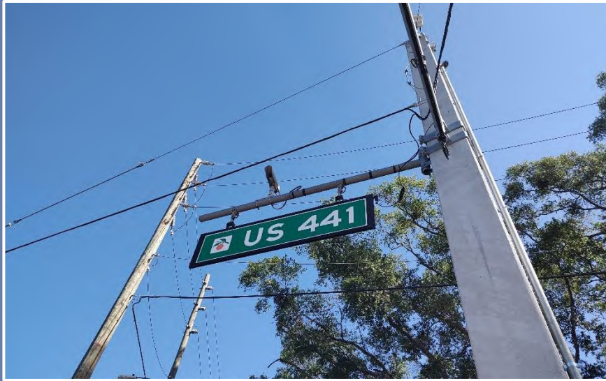
Video detection camera installed on cantilevered mounting arm for span wire intersection. (Orange County)
