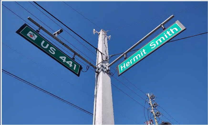
Two (2) microwave radar sensors installed directly to the concrete strain pole. (Orange County)
