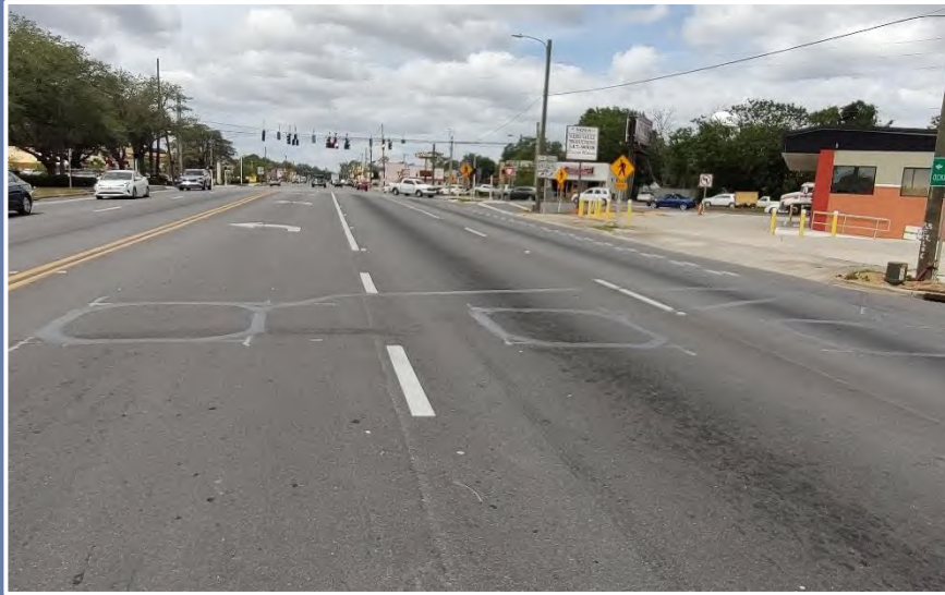
Type B inductive loops provided for advanced detection in the left turn and thru movement lanes. (Marion County)
