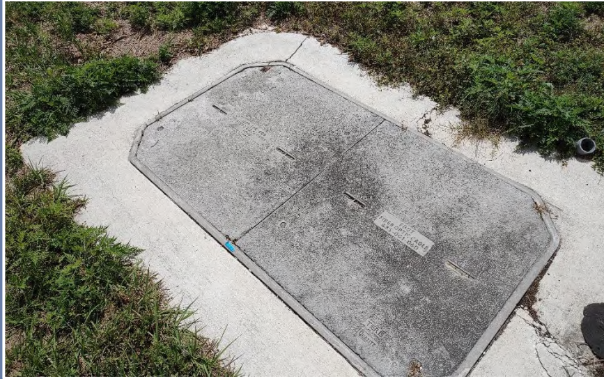
Two-section lid fiber optic splice vault (30" X 60") with concrete apron. (Marion County)
