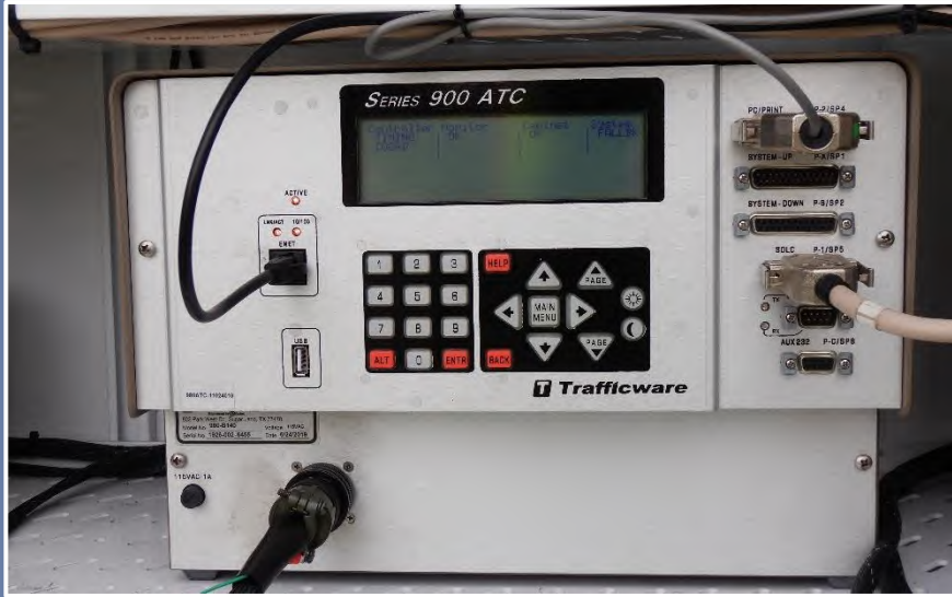
Trafficware (now Cubic ITS) 980-ATC controller unit, NEMA TS-2, Type 1 model. (Seminole County)
