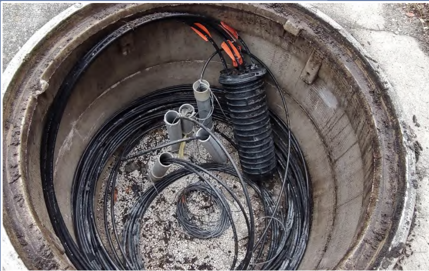
Interior of round fiber optic splice vault with conduit sweeps, cabling slack, and underground splice enclosure. (Orange County)
