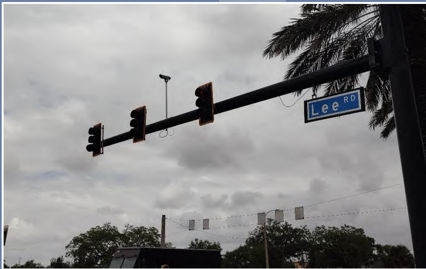
Mast arm structure with video detection camera on vertical riser mounting arm. (City of Orlando)
