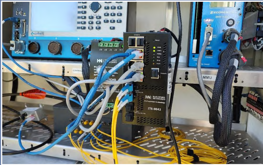
Managed field Ethernet switch and power supply installed on DIN rail rigidly affixed to the front of a shelf within the controller cabinet assembly. (Osceola County)
