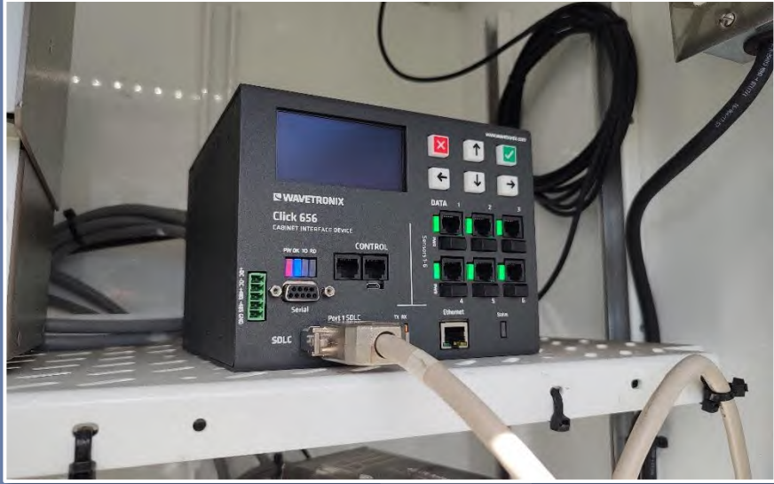
Example in-cabinet processor with capacity for six (6) unique microwave vehicle detection system sensors with SDLC bus connection. (Lake County)
