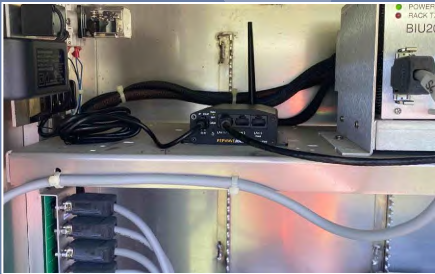
Cellular modem with embedded antenna; however, external antennas may be installed to the exterior of controller cabinet assemblies to boost signal strength, where needed. (Marion County)
