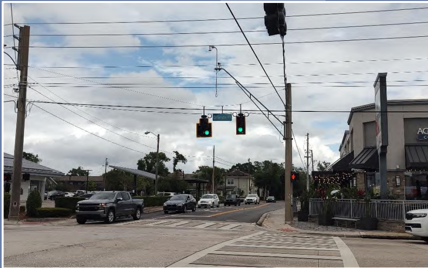
Video detection camera mounted on luminaire support arm for increased elevation above the road surface in a span wire intersection. (City of Orlando)
