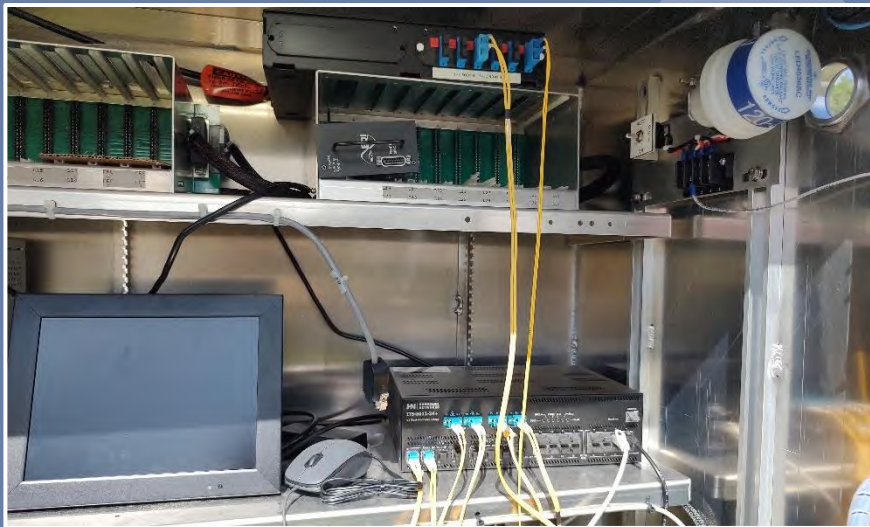
Connections between the fiber optic patch panel and the managed field Ethernet switch is developed using fiber optic jumpers; yellow for single-mode, orange for multi-mode. (Lake County)
