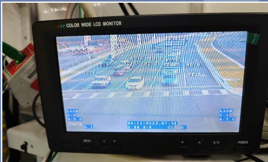
LCD color monitor installed in controller cabinet assembly displaying active vehicle calls for advanced detection zones. (Orange County)
