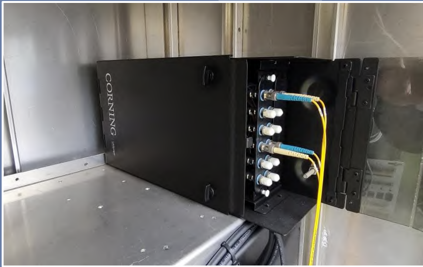
Shelf-mounted fiber optic patch panel with twelve-count connector panel. (City of Orlando)
