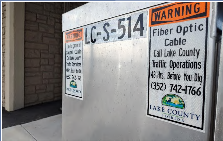
Warning label for fiber optic cable within the vicinity adhered to the outside of the controller cabinet assembly. (Lake County)
