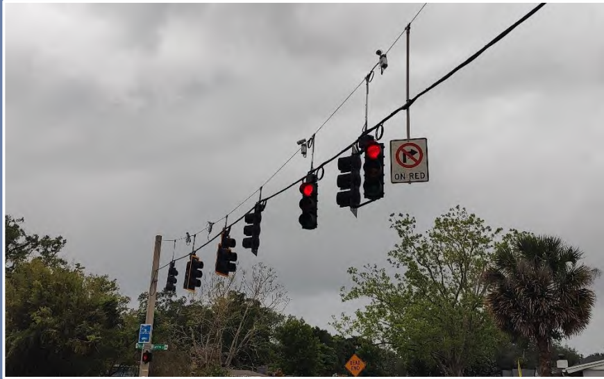
Video detection cameras installed directly to the catenary wire of a span wire intersection. (City of Orlando)
