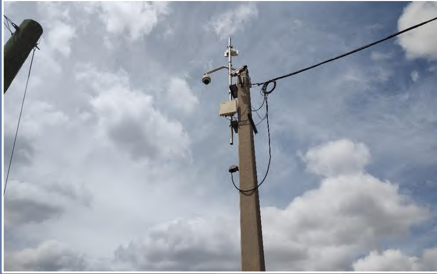
Multiple point-to-point wireless radios installed to vertical riser mounting arm creating connection between signalized intersections. (Marion County)
